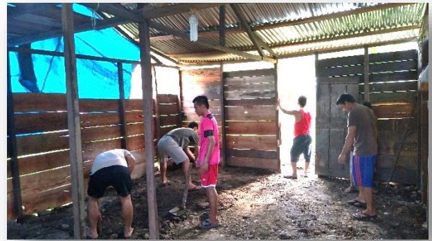
Matt and his team re-cladding and installing a concrete floor in the home of two of the scholarships students
